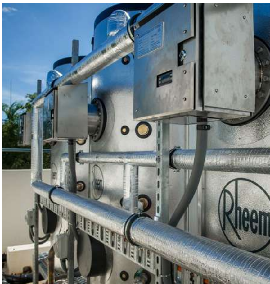
Rheem HS Series solar with electric boosting in the top of solar tanks. Katherine Hospital NT.
