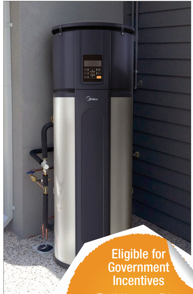
280L Installed Unit
